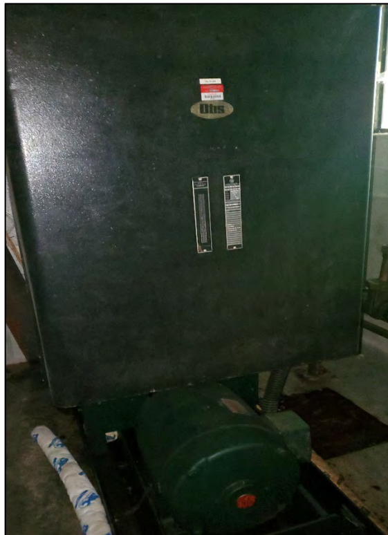
Photograph 14: View of hydraulic oil reservoir (elevator).
