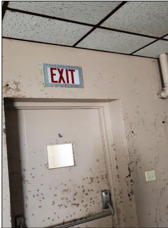
Photograph 19: View of a typical emergency exit sign.
