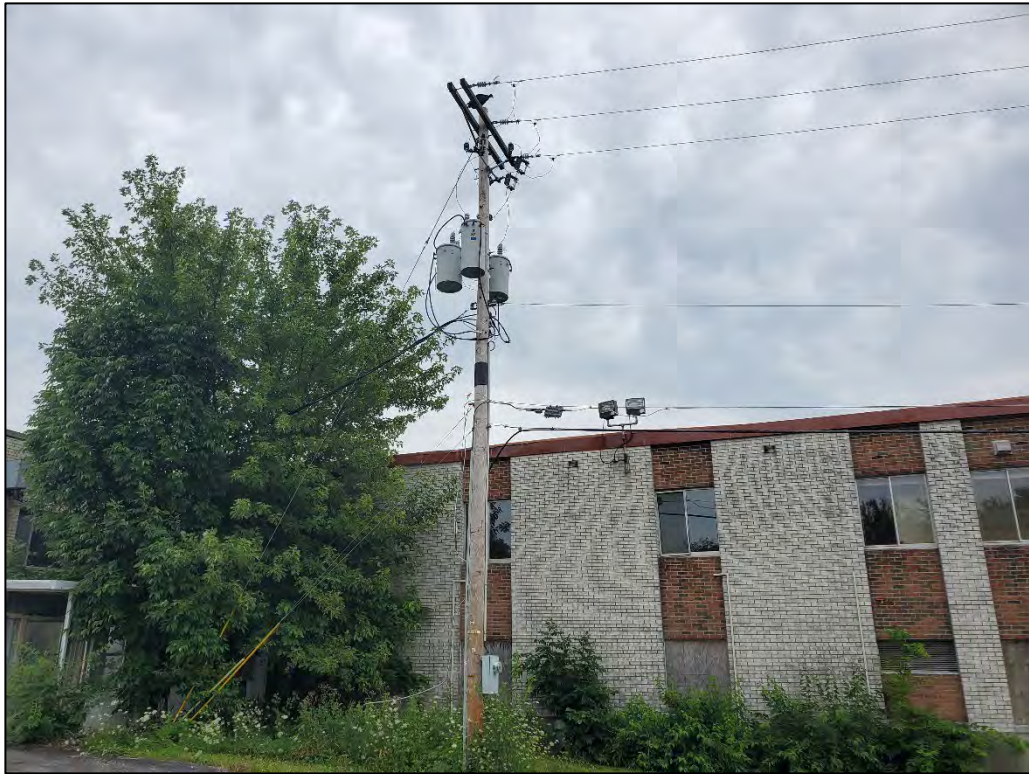
Photograph 7: View of the pole-mounted transformers located on the north side of the building.
